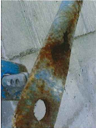
Check for scaffold damaged parts
