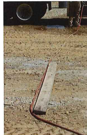
Protect water hoses from construction traffic.
